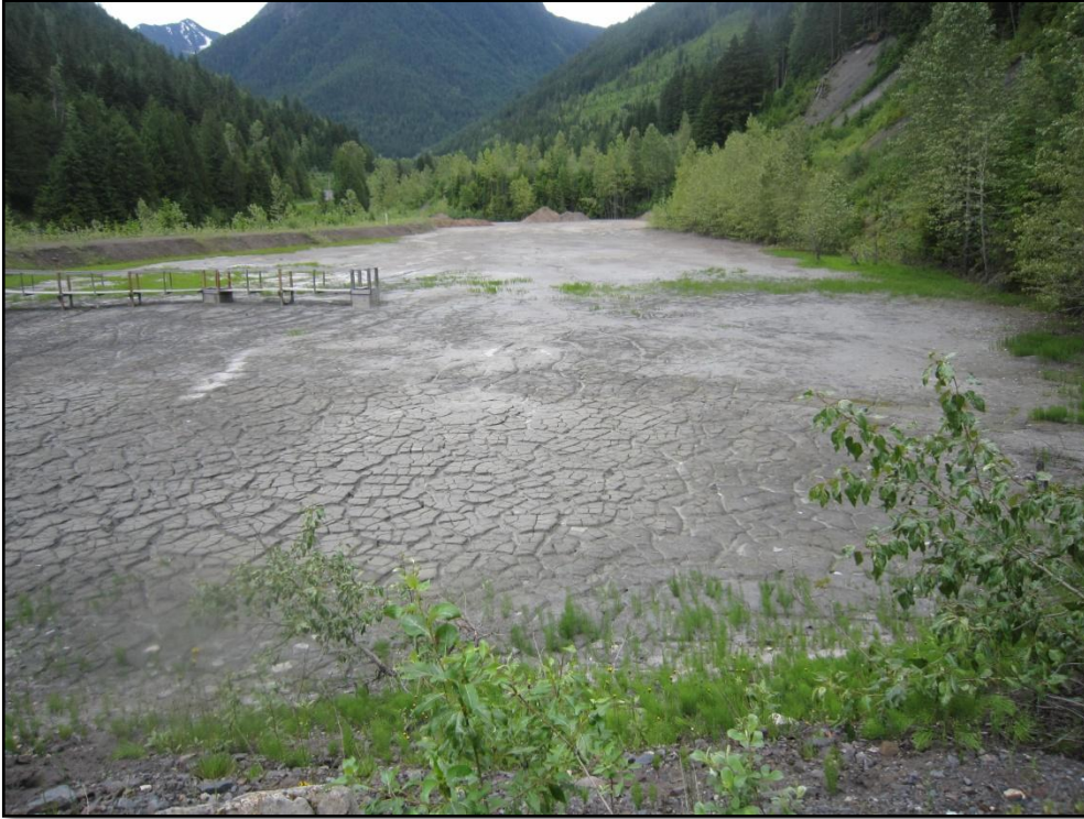
Photo 10. No. 1 pond, June, 2016; remedial work in progress includes brush clearing along the pond edges, raising the berms and dams, and adding riprap along banks of Carpenter Creek on the west side of the ponds.
